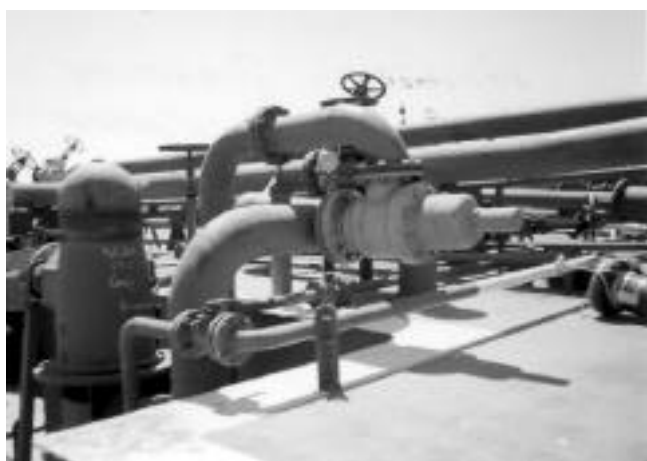
Horizontal PV Valve Installation found with trapped gasoline.
